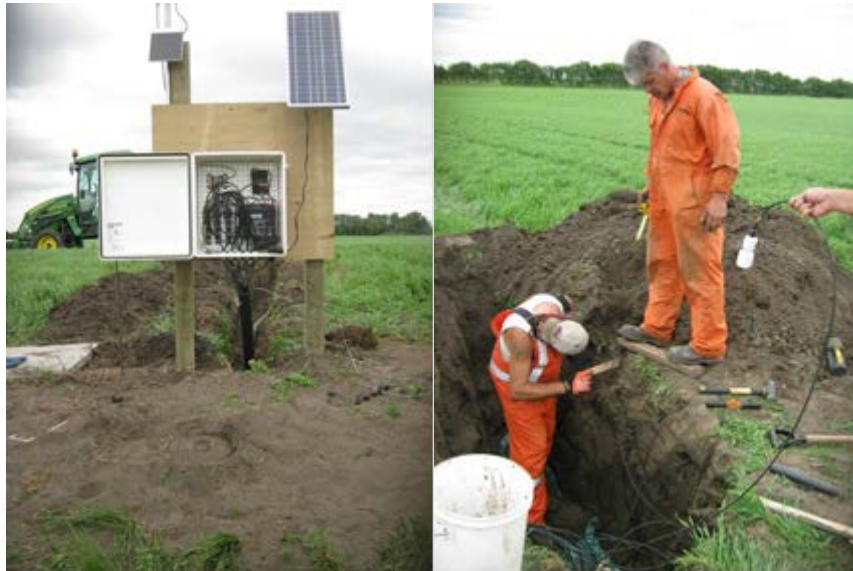
Figure 6. Site installation for AAFC in situ soil moisture sites.
